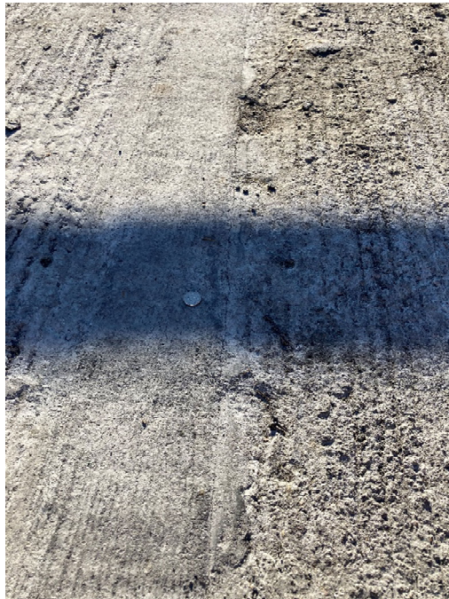
Figure 40. Crack at interface of UHPC joint and precast deck panel on Span 2 (quarter provided for scale)
