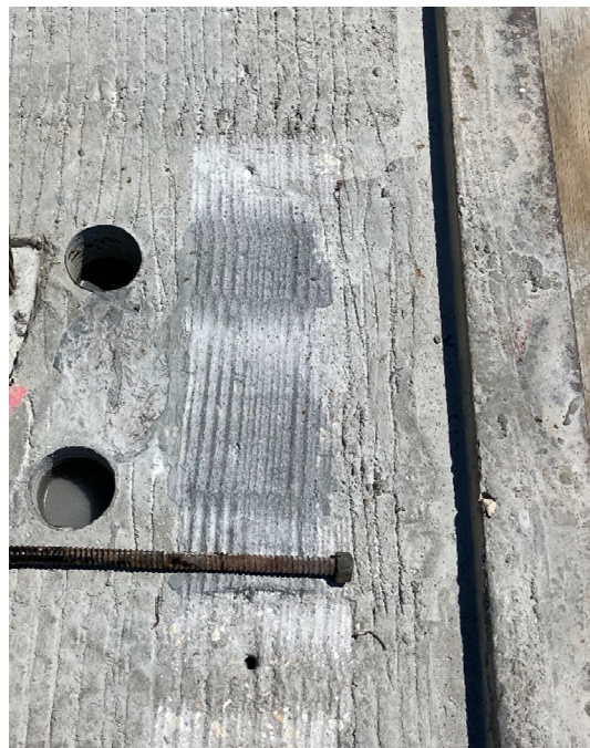
Figure 13. Close-up view of ground UHPC shear pocket to show texture after grinding
