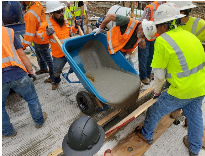
Figure 9. Placement of UHPC into transverse deck joints of the mock-up and flow “uphill” under the head pressure of the material. Once the joint was nearly full a form top was placed on a section of the joint and attached to the deck using concrete screw anchors. The placement point was then moved along the joint. Buckets with holes in their bottoms were connected to holes in the top form at approximately 8 ft intervals along the joint length and UHPC was added to these buckets to maintain head pressure on the UHPC in the formwork (Figure 10). The material was allowed to flow along the
