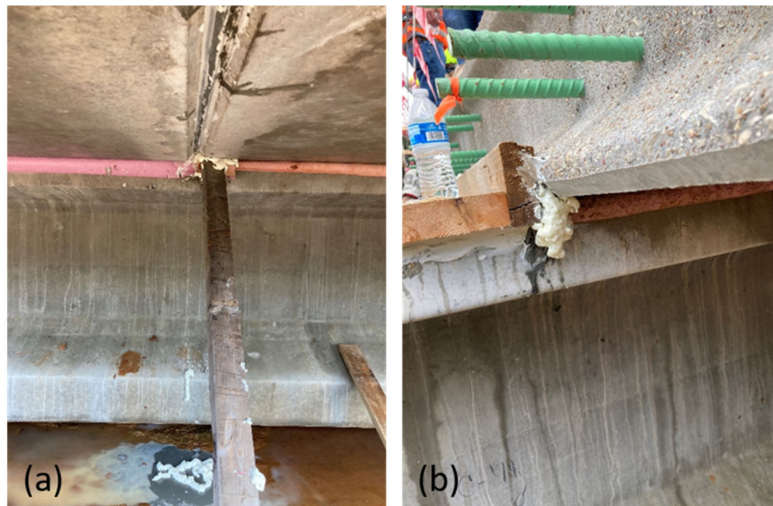
Figure 11. Bracing and spray foam utilized to stop a leak at a (a) deck joint to girder intersection and (b) end of the haunch
