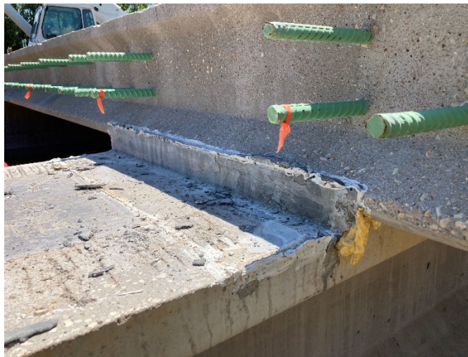
Figure 16. Photo of the end of the UHPC haunch showing that the forms were filled at the farthest location from the placement points
