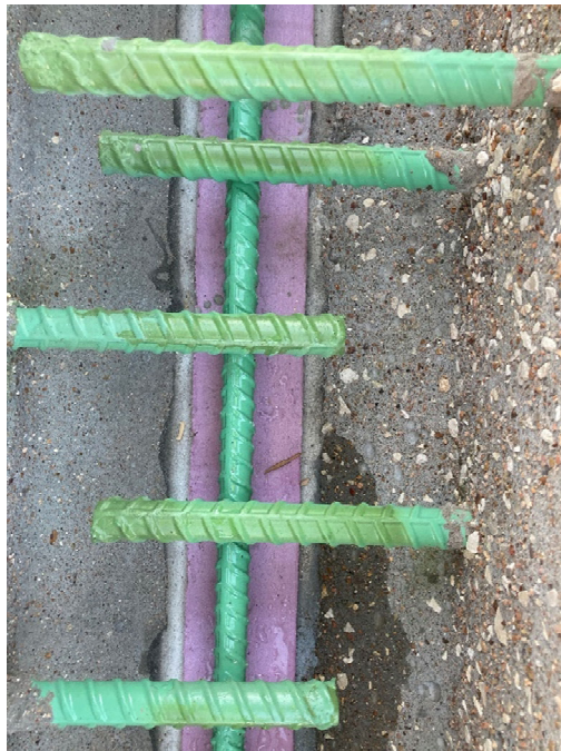
Figure 34. Insulation foam and cementitious grout used to seal the bottom of the joint
