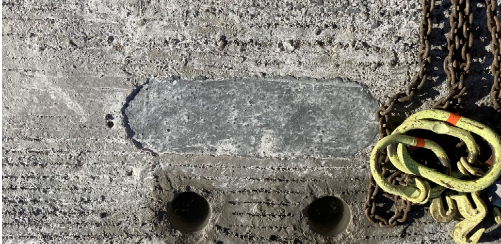
Figure 41. Shear pocket that was not filled above the level of the top of the deck
