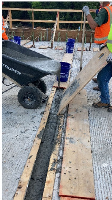
Figure 10. Top formwork placed on completed UHPC placement and head buckets in place
