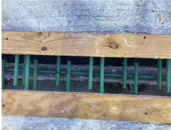
Figure 27. Foam insulation and caulk used to seal the bottom of the joint
