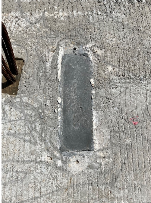
Figure 15. Close-up view of a shear pocket where the UHPC did not extend above the top of the slab as intended
