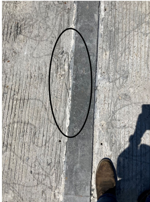
Figure 14. Crack alongside UHPC joint caused by formwork anchors
