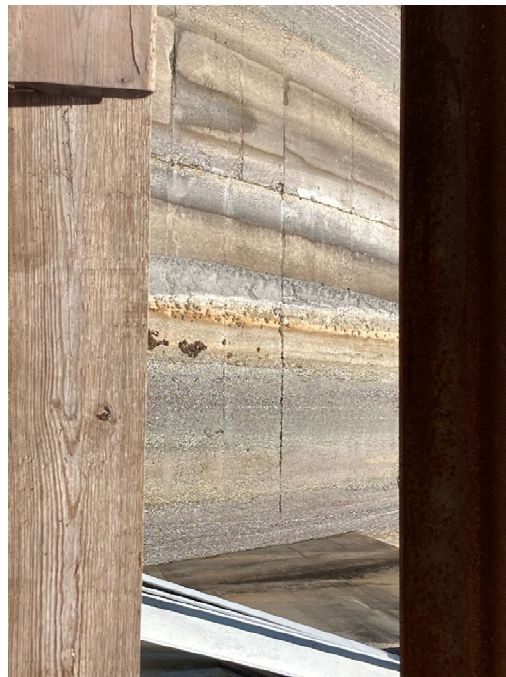
Figure 37. UHPC material from formwork blowout remaining on concrete spillway channel
