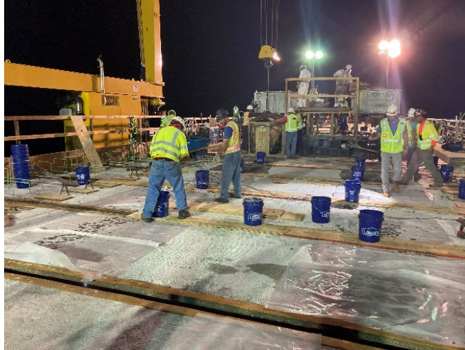
Figure 29. Concrete mixers used on the bridge placements with one mixer being discharged into the concrete transfer bucket. Head buckets in place on the joint top forms are also visible
