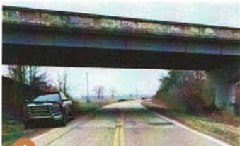
1 State Route 88 was in poor condition
