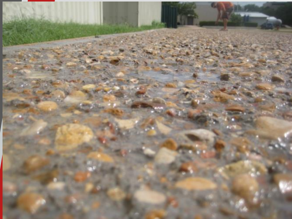
Abraded Concrete Surface
