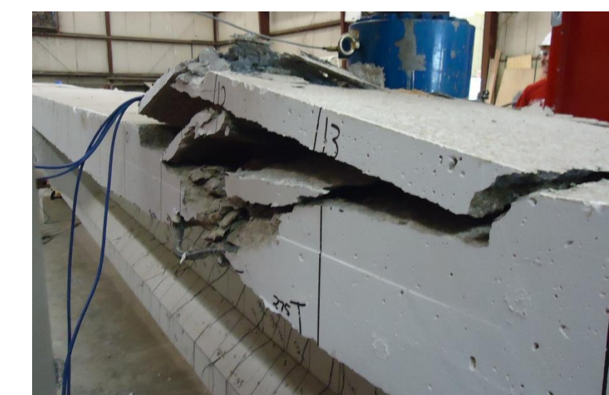
Damage from Initial North End Testing, East Side (Above)
