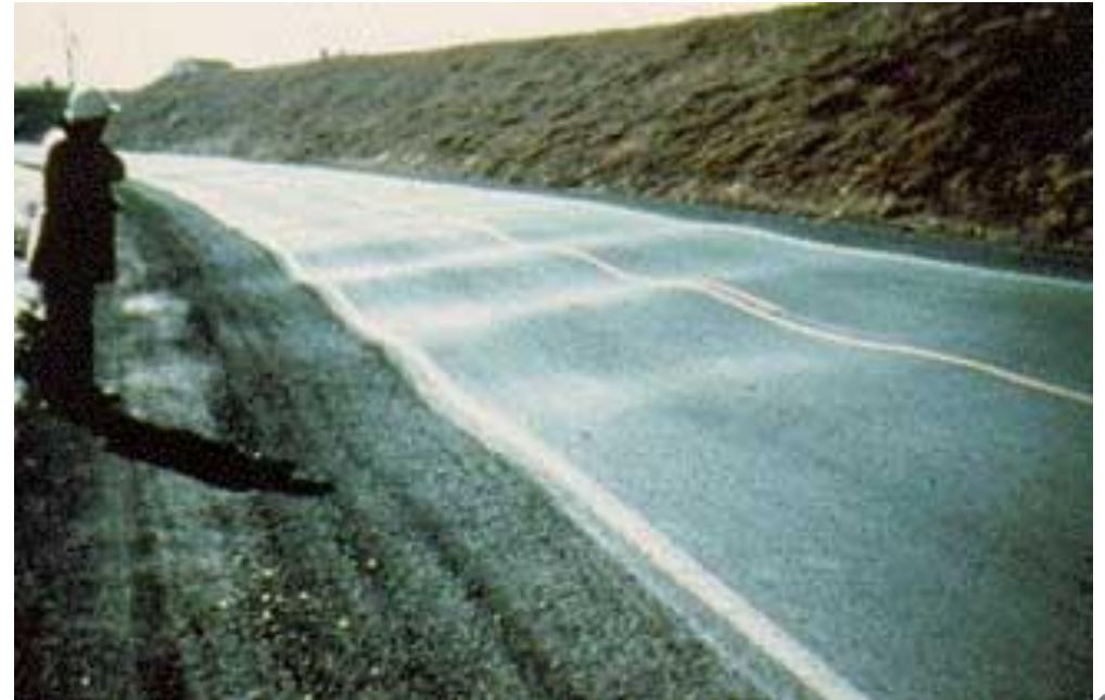
Distortion due to frost heave
