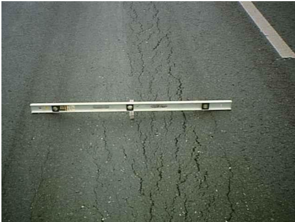
Rutting due to unstable subgrade
