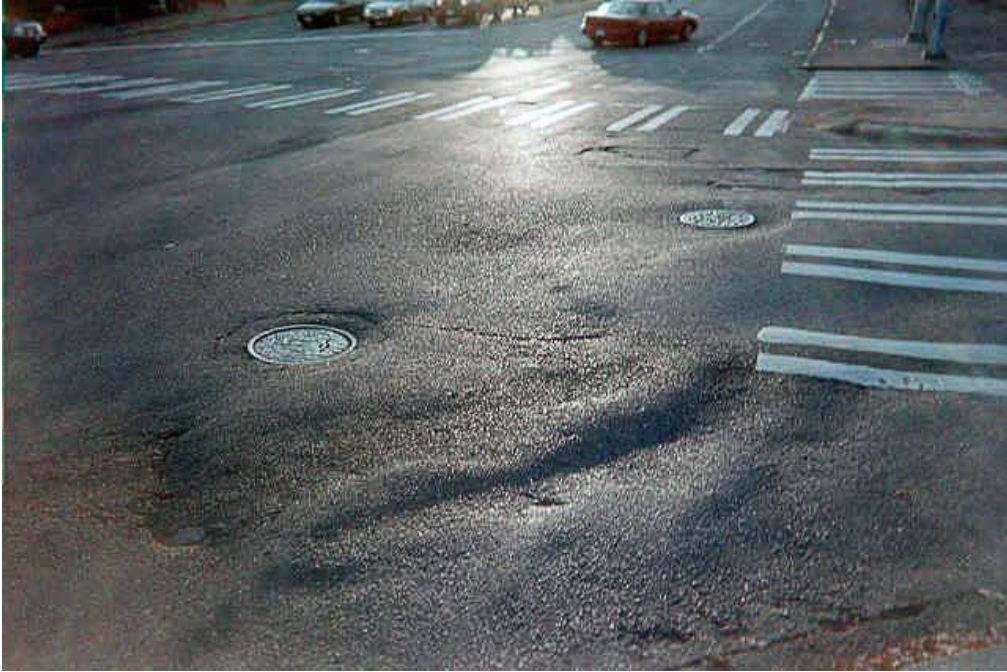
Corrugations and shoving
