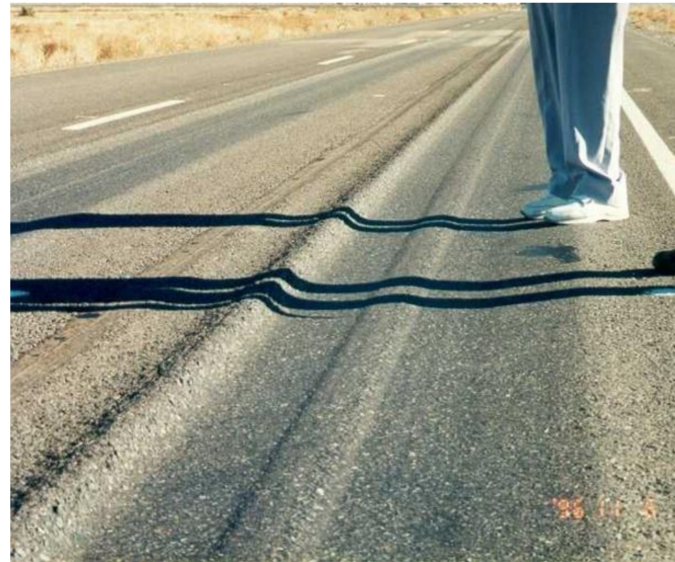
Rutting due to unstable plastic mix
