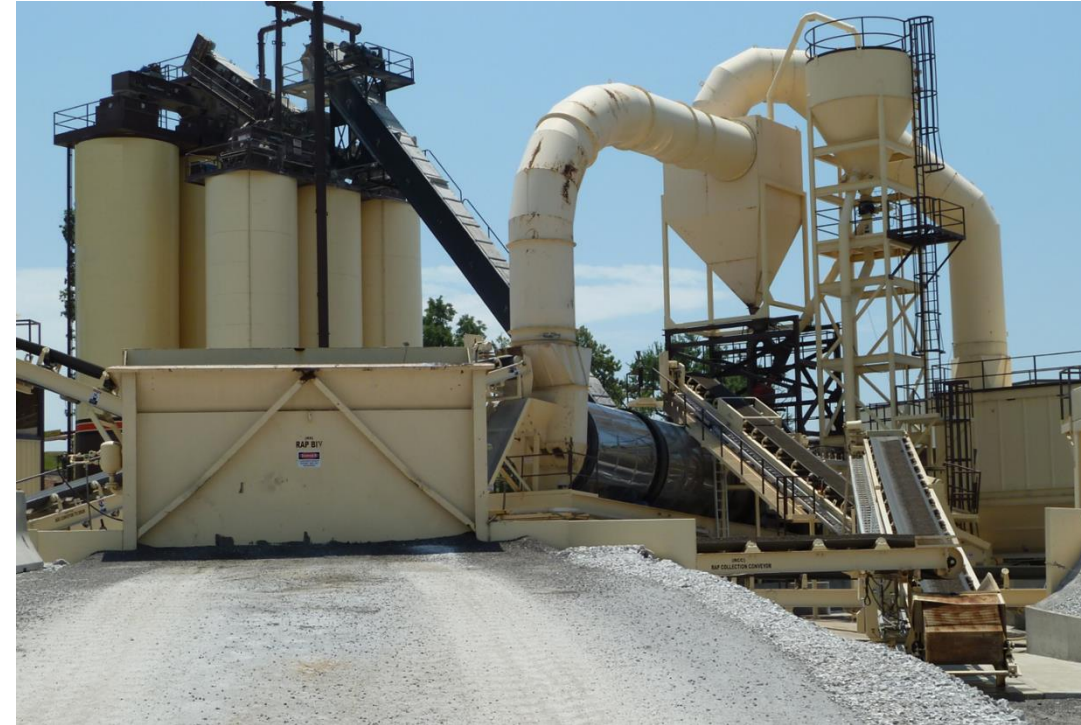
An asphalt mixture plant in NWA
